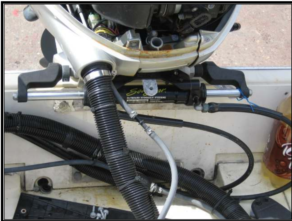
SEA STAR steering system does not appear to be damaged
