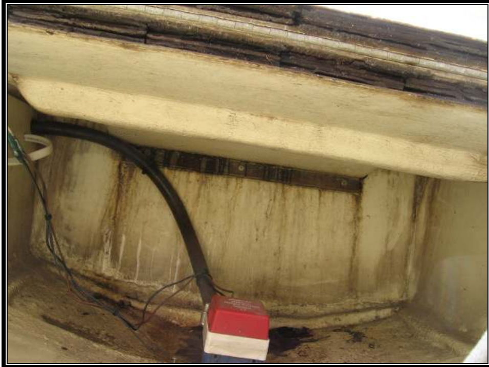
Failed bilge pump with float switch; Note the stains on the transom indicating leakage over time.
