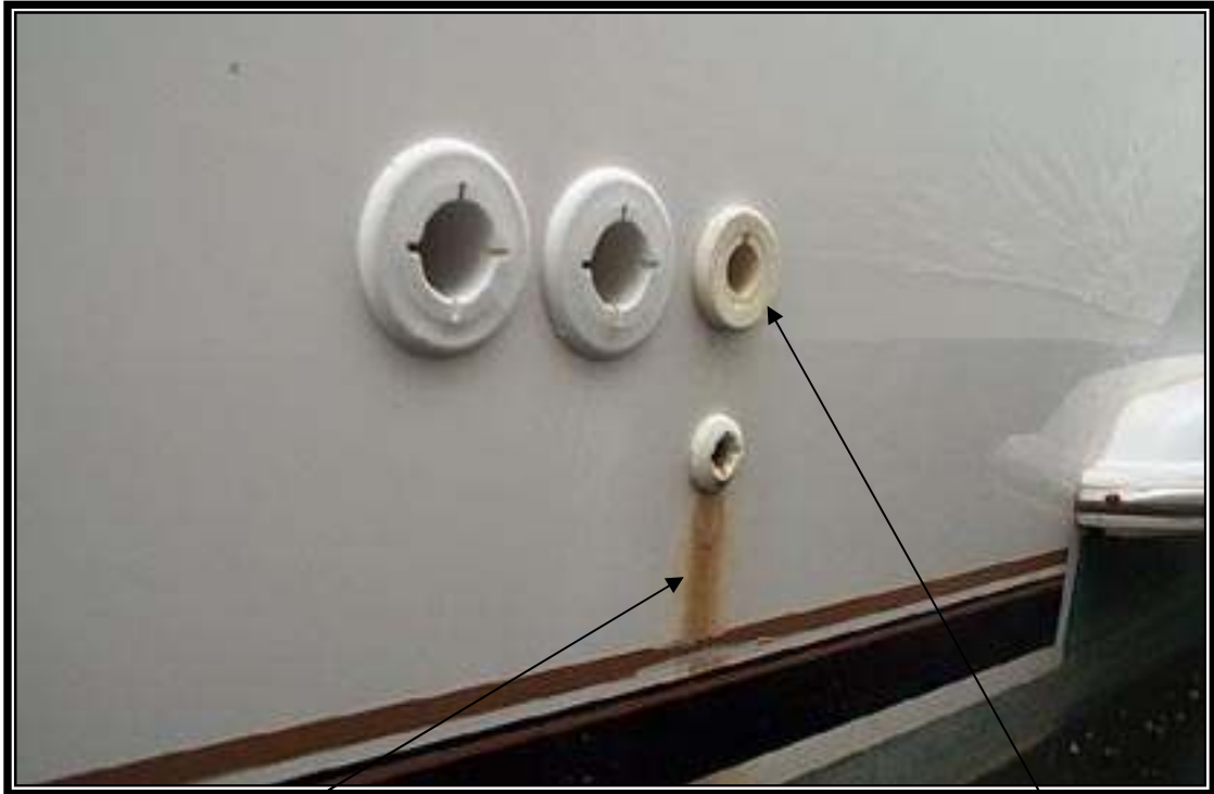
Discoloration at Portside Drain – Through-Hull Showing UV Deterioration
