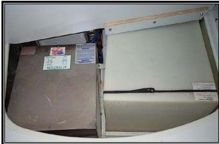
Water Heater & Water Tank
