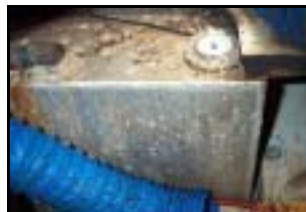
Corroded/leaking Fuel Tank
